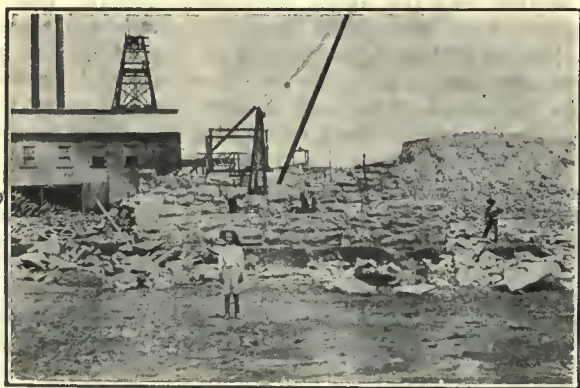
FOUNDATIONS FOR NEW CONCENTRATOR AT NO. 4 SHAFT AT THE MESSINA COPPER MINE.
